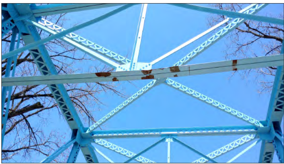
Here is the damage seen at the top of the 300W bridge over the Wabash River south of Ind. 116. The Wells County Commissioners reviewed the damage Monday via pictures. (Photo provided)
