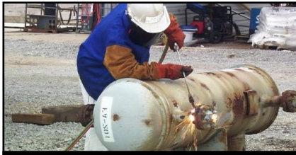
Newport_FPF_8 Newport demolition recovered more than 5 million pounds of metal. A worker at the Newport VX Production Facility at Newport Chemical Depot, Ind. cuts a length of decontaminated pipe removed from the facility. The U.S. Army recycled more than five millions pounds of scrap metal from the facility's demolition.
