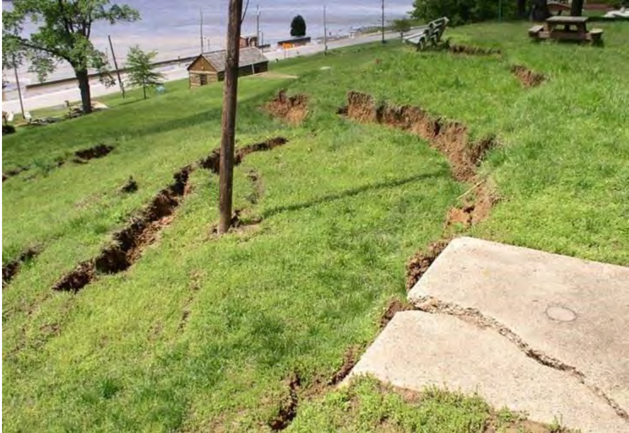
Figure 145. Newburgh Landslide Prior to Mitigation
