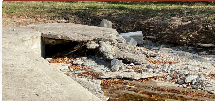
September flood in Switzerland County damages culvert and roadway
